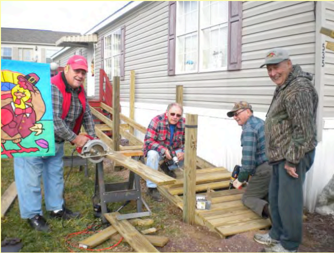
Lions John Weist, Dwight Kutz, Bruce Altland and friend Marty Smith building a ramp for Lion Cathey Stump at Rich and Cathey's home
